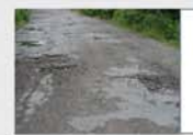
Bell Rock Rd crossing Queen Gutter Brook near Wilson Rd. Unpassable Road Conditions. 3
