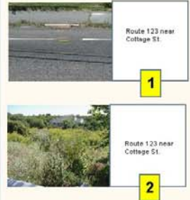
Route 123 near Cottage St; an all culvert under road drains directly into channel through lush wetland near new development. Evidence of mosquito ditching. This site may retain stormwater during peak flows. Larger culvert may be necessary here.
