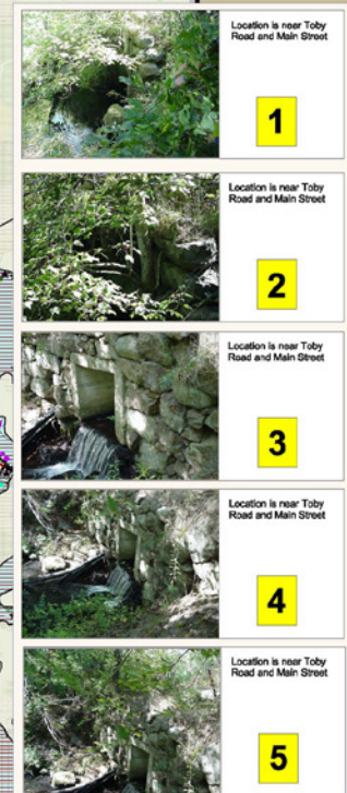
Deteriorating stone headwall and concrete box culvert; stone loose in spots with vegetation growing out of the headwall, including a large caliper tree on the north side of the street; several black 6" corrugated plastic hoses through the base of the headwall on the south side of the street (upgradient from what appears to be a homemade fisheries operation/run of some sort).
