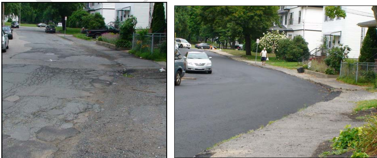
Figure 8-3: Poor Conditions with Improvements
